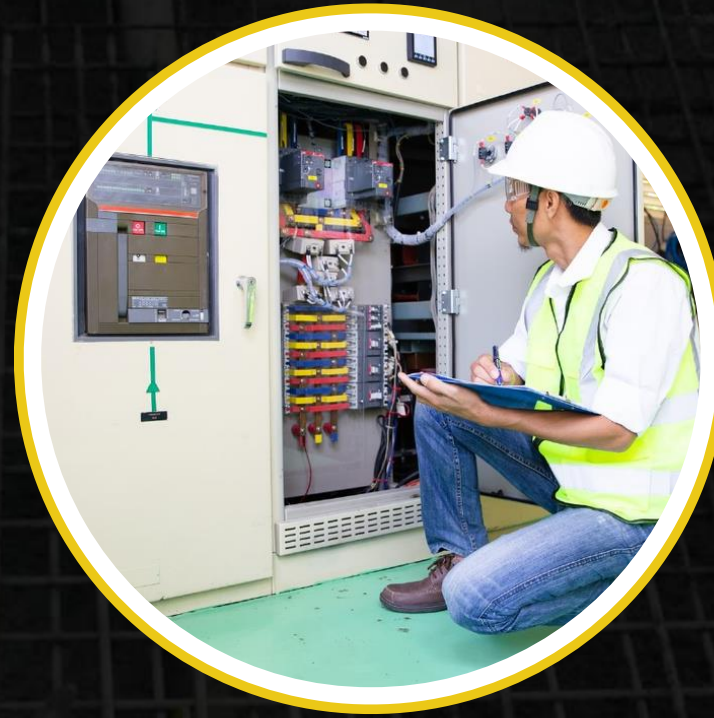
Electric And Telecom
